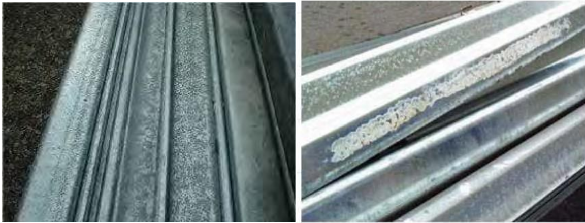
Fig. 8 Formation of white rust in the Zinc galvanized coated CFS members
