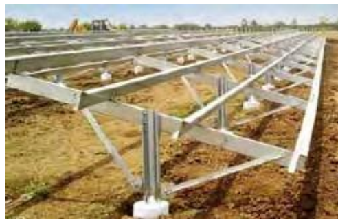
CFS members in solar mounting frame
