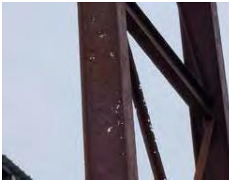
Pitting corrosion of steel columns in a detergent manufacturing plant due to the presence of salt and active matter.
