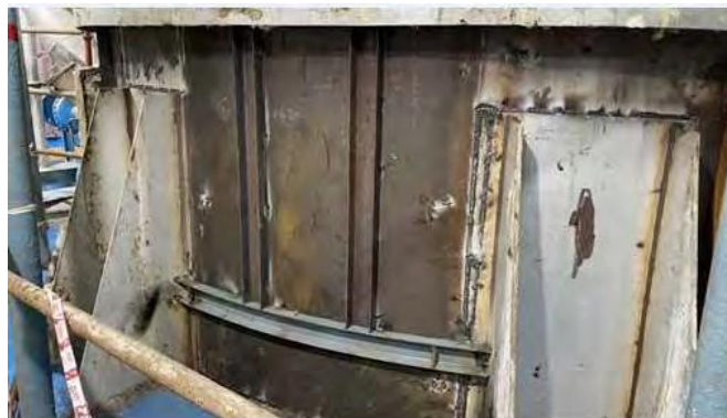
Pictures of corrosion of spray drying tower
