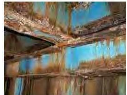
Crevice corrosion in beams
