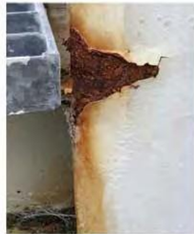
Galvanic corrosion due to different anodic index between the bolt and a plate
