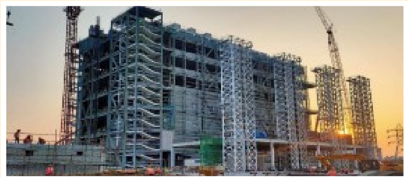
Fig 23 : AdaniConneX Centre, Chennai
